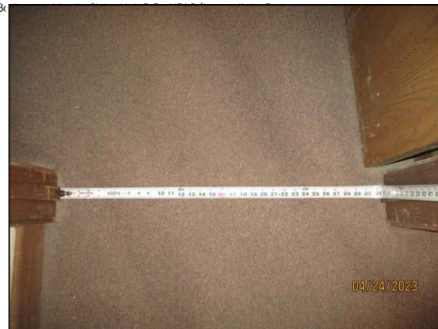
99 : Narrow Bedroom Door Opening Width - Unit B-9 - UFAS (Immediate Repair)
