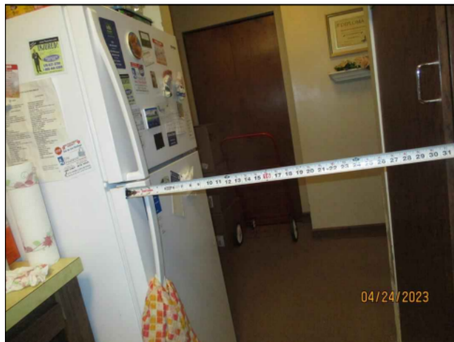
Clear Floor Space at Accessible Unit L-Shape Kitchen - Unit B-11 - UFAS (Immediate Repair)
