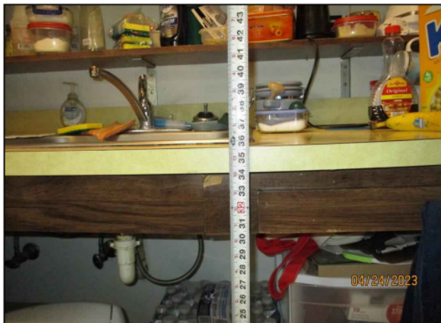
Compliant Height at Roll-Under Kitchen Sink with No Scald and Abrasion Protection - Ur
