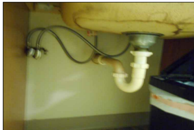
ated handicapped dwelling units do not feature scald and abrasion protection at plumbing (Immediate Repair)
