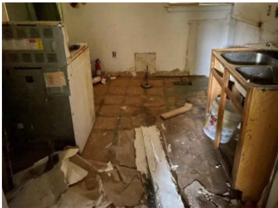
4. Down dwelling unit (Critical)
