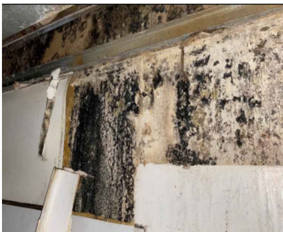
Down dwelling unit (Critical)
