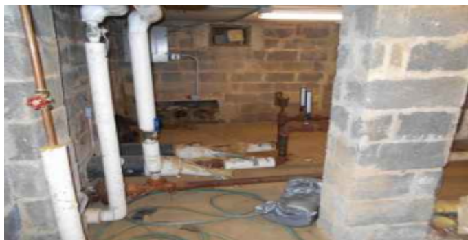
9. Copper supply piping
