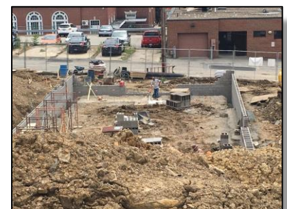
Construction continues as City Mission expands its facilities with housing for veterans.
